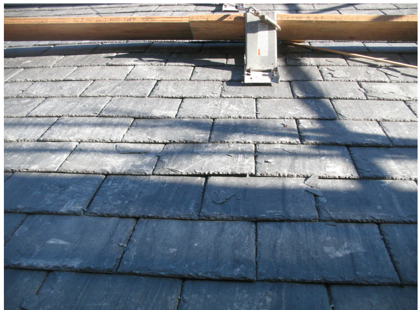
Figure 2: Slate fines and fragments present on the roof prior to the final sweeping-down. Some of these will invariably remain on the roof and gradually get washed down into the gutters with each passing rain.
