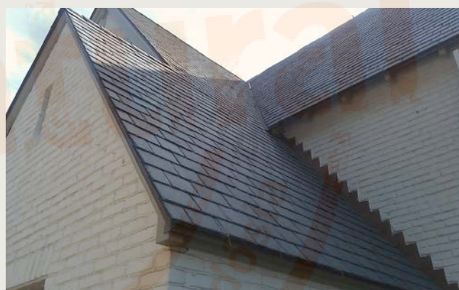
Nails roofing system
